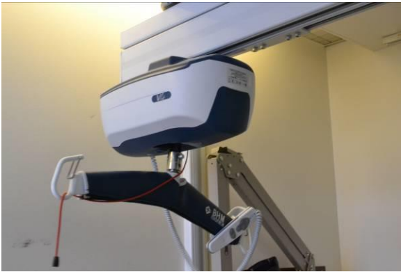
Room 514 Ceiling Lift
