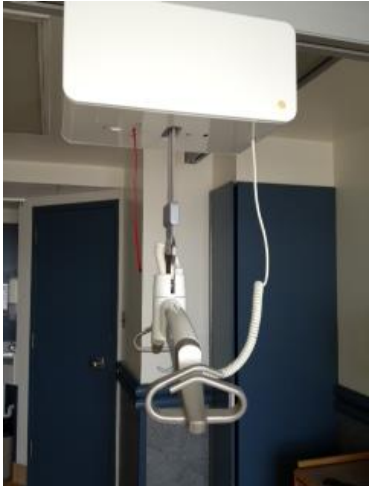
Bariatric Ceiling Lift Rm 218
